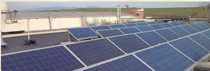
Installations in industries and commercial buildings
