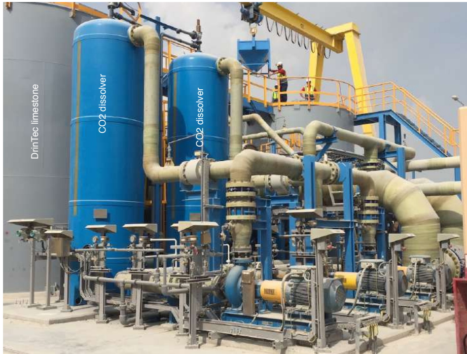
Fig. 10: Two CO 2 dissolvers measuring 1.4 m in diameter and 5 m in height at the inlet of a DrinTec™ remineralisation plant. Photo courtesy of Acciona Agua.
