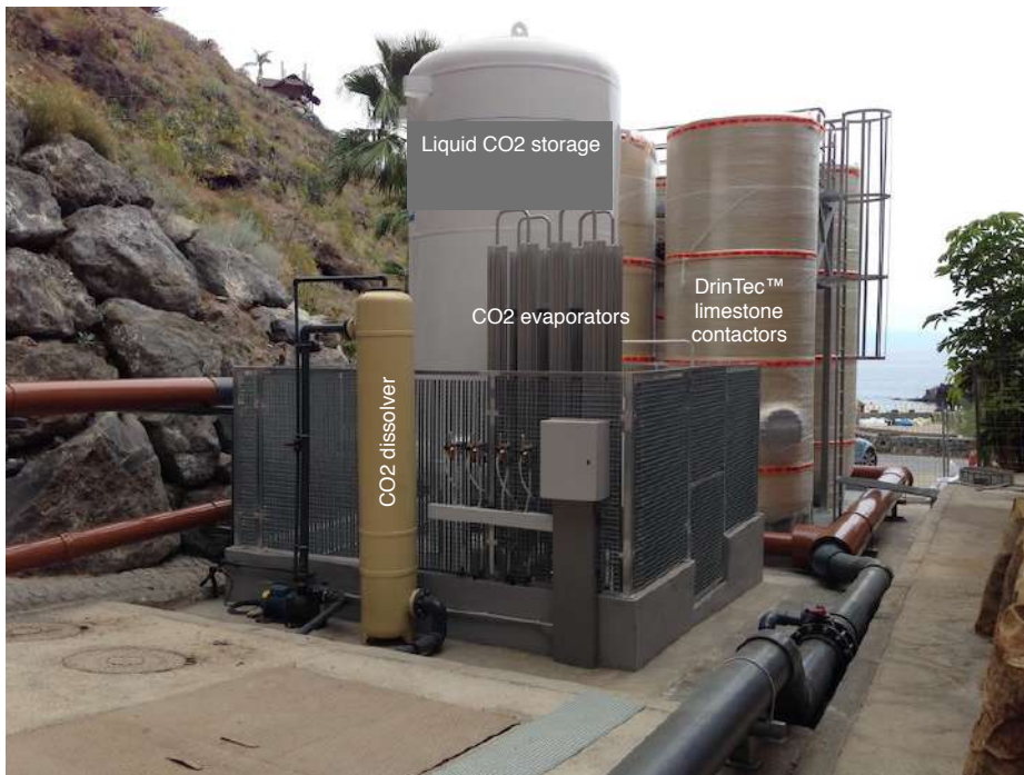
Fig. 11: CO 2 dissolver in bypass configuration at the inlet of a remineralisation plant with DrinTec contactors. Photo courtesy of Tagua, S.L., Canary Islands.
