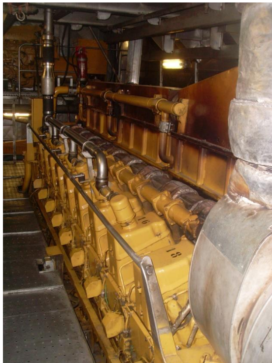
Fig. 14. Vista del motor principal SOME
