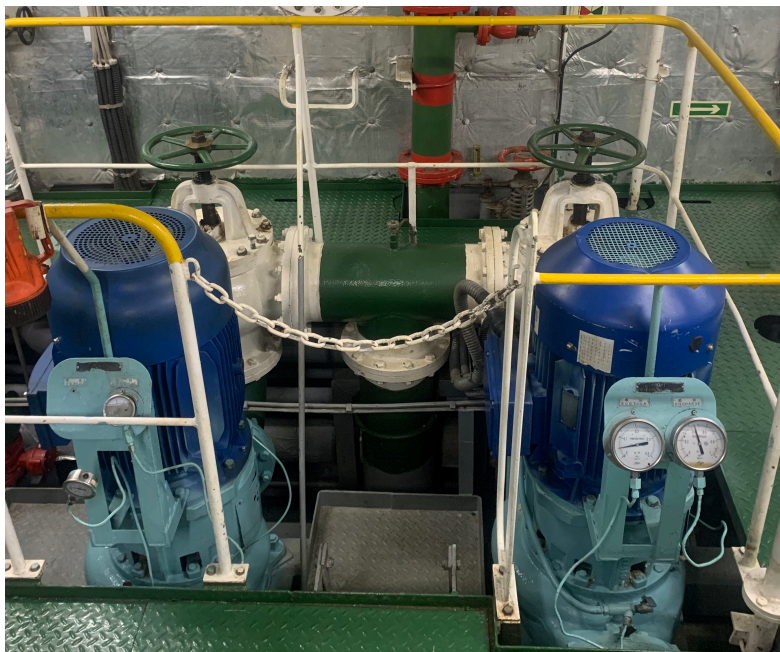
Ilustración 7: "Bomba vertical centrífuga AS buque Tinerfe"
