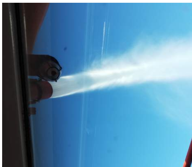
FIGURA 2.2: Monitor contraincendios babor. (E. Arévalo 2020)
