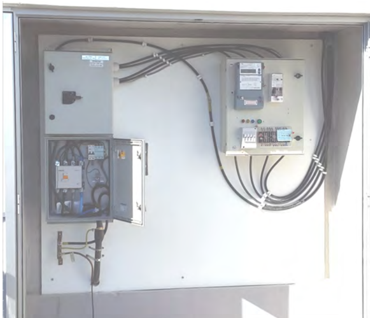
Figure 4.20: Electrical switchgear detail for self-production PV system
