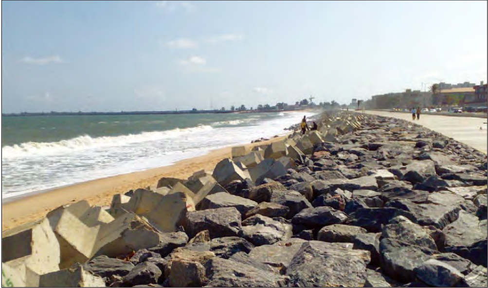
Figure 1.19: Bar Beach seawall, Victoria Island, Lagos, Nigeria
